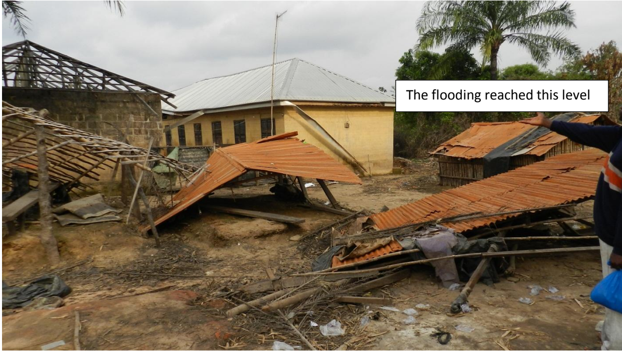
Figure 12 Rusty roofing sheet telling the story of the severity of the flooding when all these structures were submerged in water
